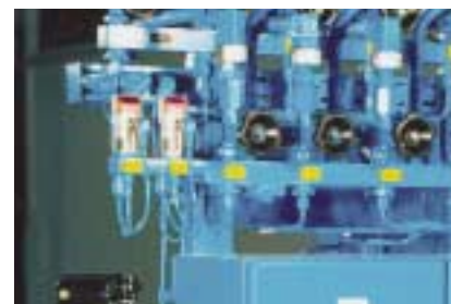
Imperative: Temperature detection in heating and air conditioning.
