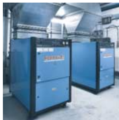
Optimised consumption of compressed air.
