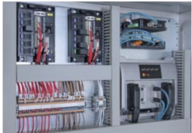
ifm's ecomatController for mobile applications (bottom right) is mounted in the control cabinet outside the vehicle.
