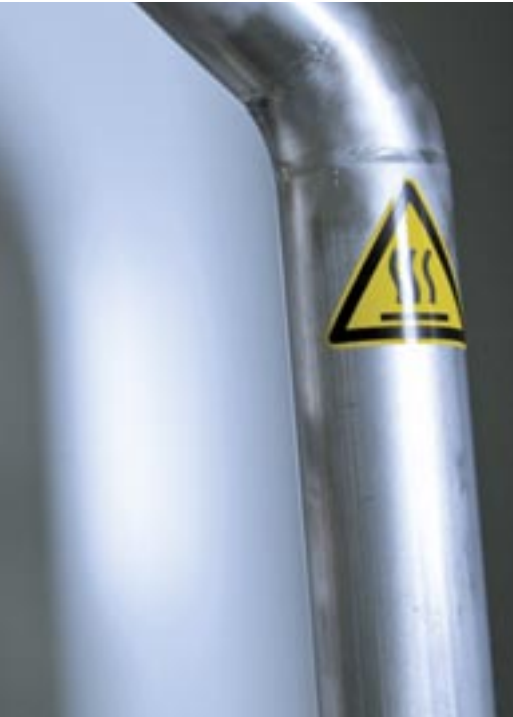
The SD9000 from ifm monitors flow and temperature of the cleaning liquid.
