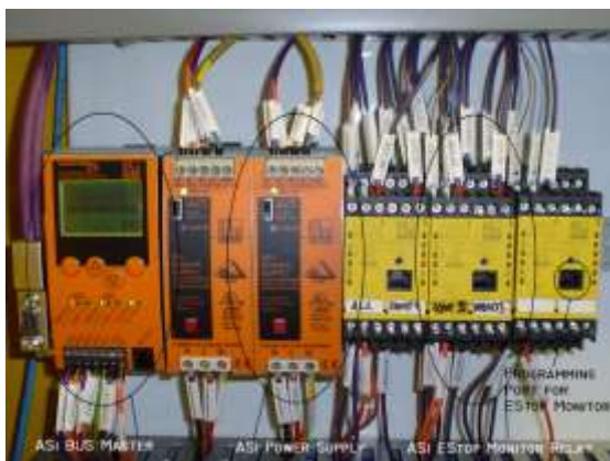
Figure 3: Controller, power supplies, safety monitor
