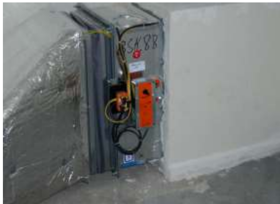
Figure 2: channel with fire protection housing
