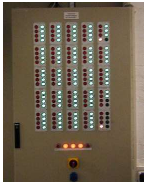
Figure 4: panel with illuminated push-buttons for each damper
