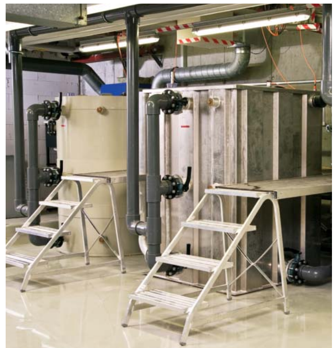
Level measurement in a water treatment plant
