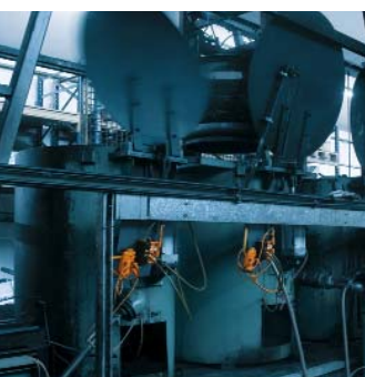
CompactLine used in a hardening shop.
