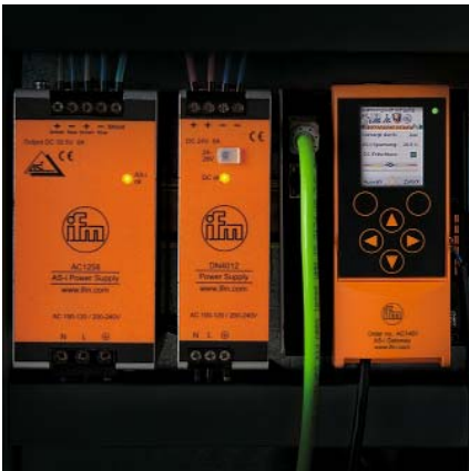
Tidy control cabinet: The central control components of the AS-i network.
