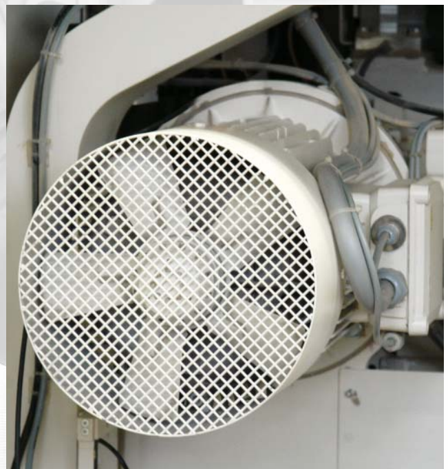
Monitoring of the overall vibration of rotating components (fans, centrifuges etc.).
