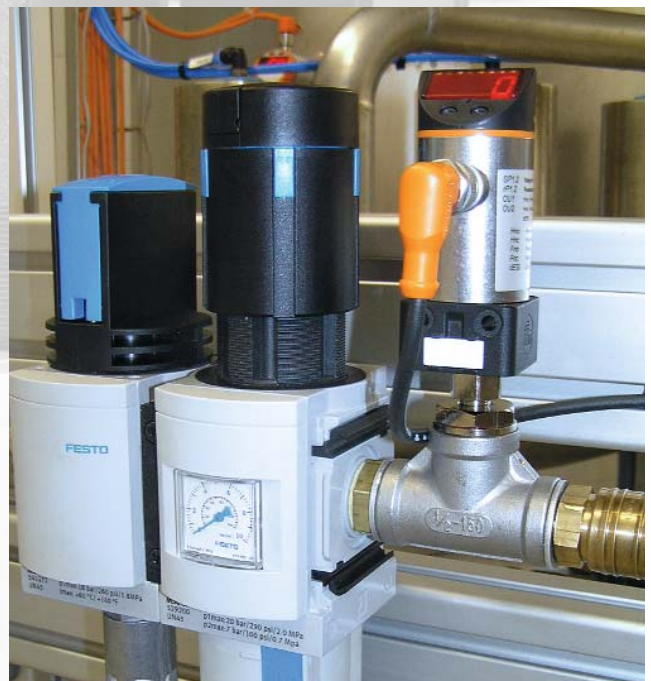
PN78 and accessories connected to a pneumatic maintenance system
