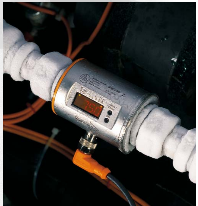
Magnetic-inductive flow sensor in water cycle for quantity monitoring.
