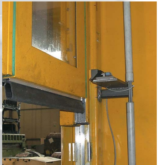
Application: Sliding door at a metal press.
